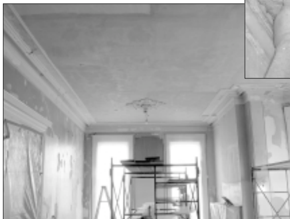
(above) Delicate repair of the plaster cornice. (left) The expansive Parlor ceiling in the midst of plastering.
